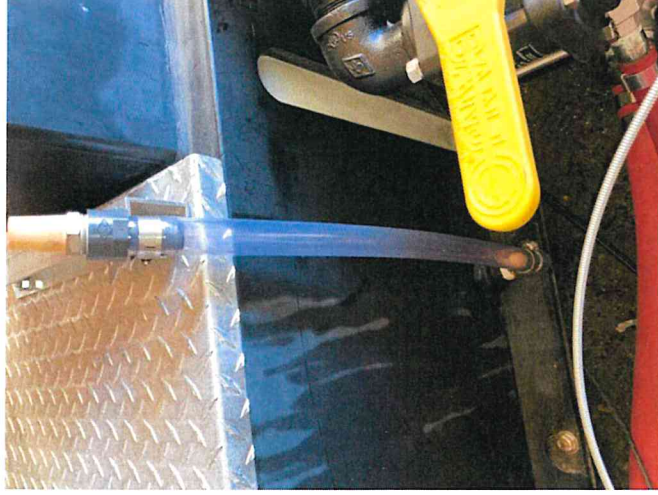
Water level site gauge, original window is no longer translucent
